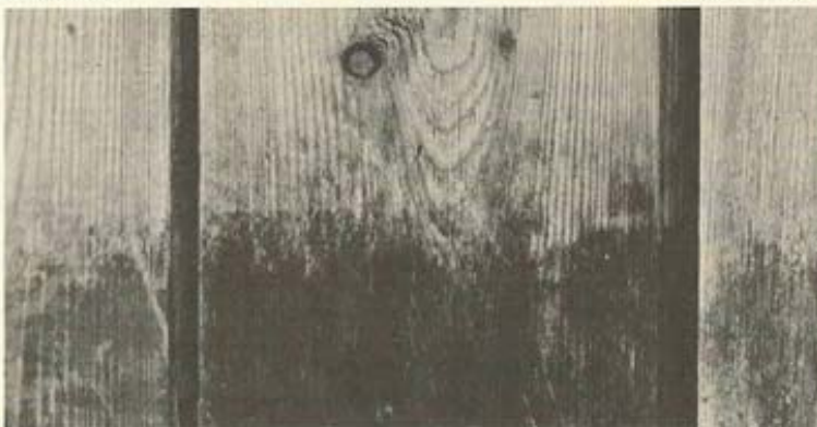
Mildew must be removed before re-finishing.
